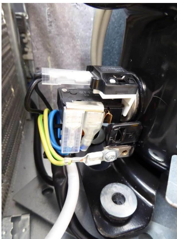
Motor start relay in position
