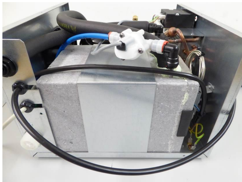
Cool water storage
